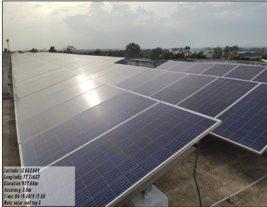
Roof-Top Solar Plant
